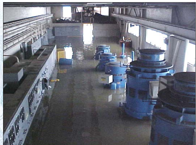
SUBMERGED PUMP MOTORS AND CIRCUIT PANELS AT EAST BANK WASTEWATER TREATMENT PLANT
